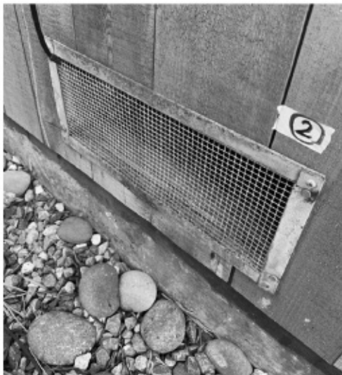
DEFINITELY NEEDS REPLACING!!!
